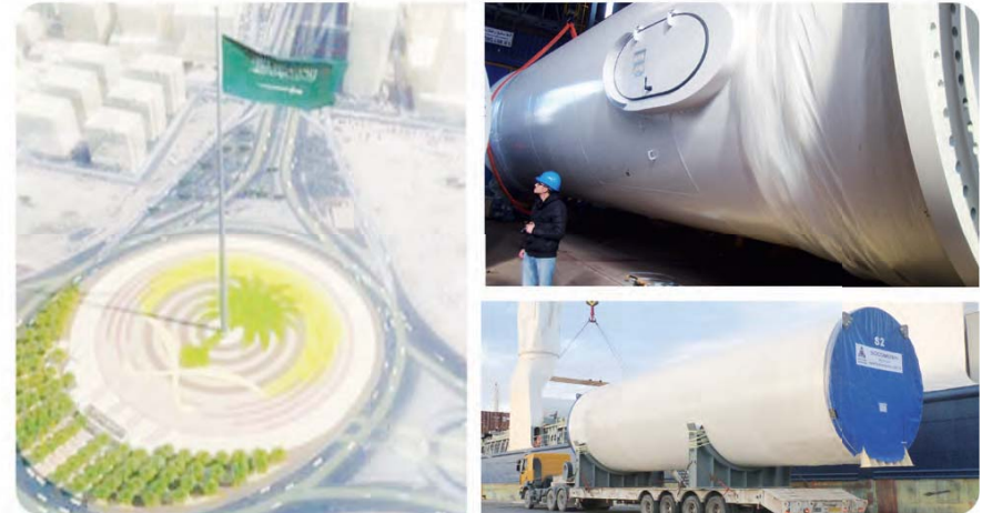
Project: Supply and Fabrication of The tallest flagpole in the world (H:170 m, Diam from 2,3 m to 4 m) located at Jeddah, KSA Main contractor: Al Babtain-Le Blanc Owner: Abdul Latif Jameel Year: 2013 / 2014
